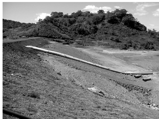
Figure 2. Emergency berm constructed along the downstream face of the Phase II dam following slope failure.
