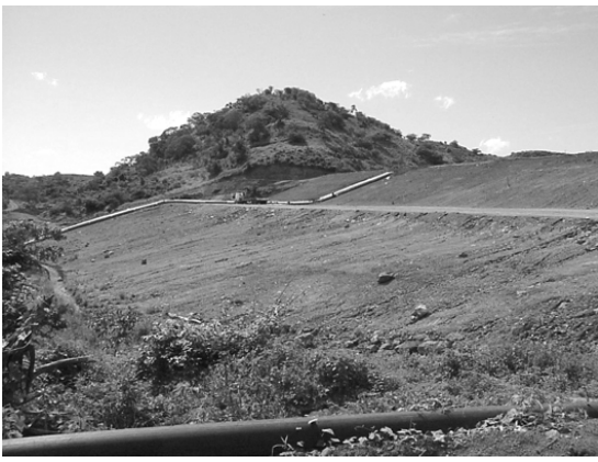
Figure 3. Cerro Santa Rosa tailings dam following construction of the Phase III downstream crest raise.
