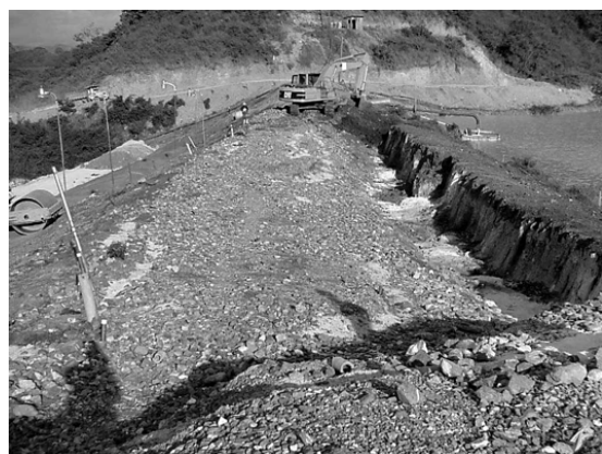
Figure 1. Slope failure scarp along the Phase II crest of the Cerro Santa Rosa tailings dam
