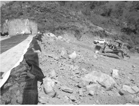
Figure 12. The downstream rockfill shell was raised at the same rate as the MSE wall.
