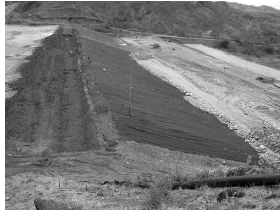
Figure 10. Construction of the sand blanket drain and downstream rockfill shell were completed as parallel tasks.
