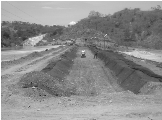
Figure 11. MSE wall construction began on 01 May 2004 with the first lift keyed into the Phase III crest.
